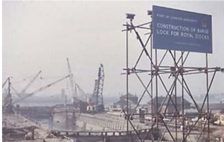
Work gets under way with heavy lift derricks and heavy piling rigs
