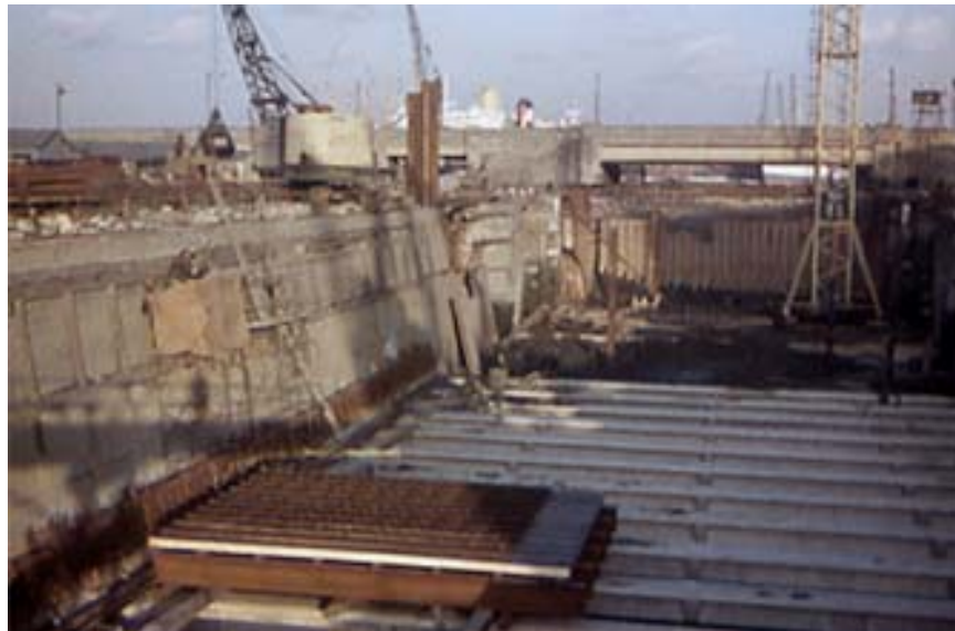
The lock has been "de-watered", and the sides supported by temporary concrete "struts". In the foreground is a large form being prepared for the first concrete pour to the new lock side walls
