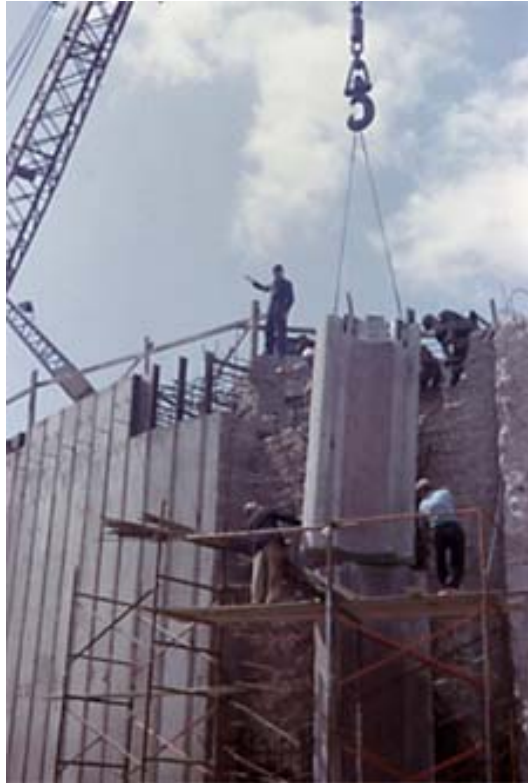
Pre-cast concrete lock gate hinge receptacle units being lowered into position. Length approx. 11' 6", weight 5 tons, required in-place accuracy of internal curved surface +/- 1/32 inch. Total height of gate quoin, 38 ft.
