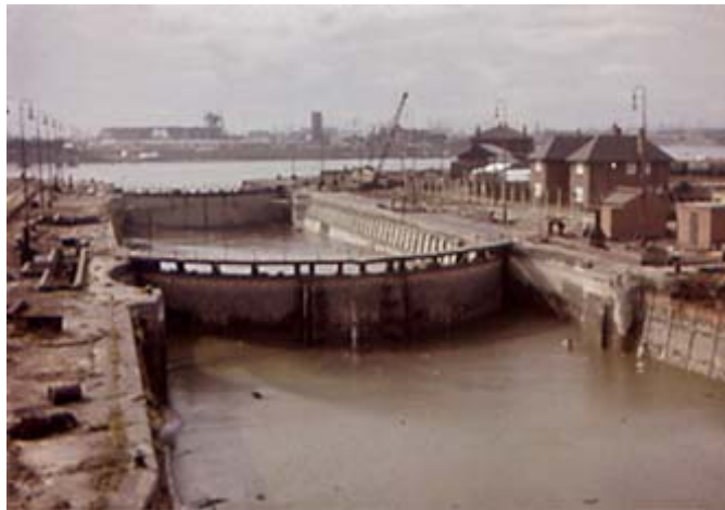
View of long-abandoned Western Entrance to RV docks prior to start of contract
